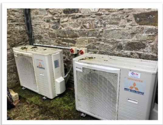
Fig 2. Air Source Heat Pumps
