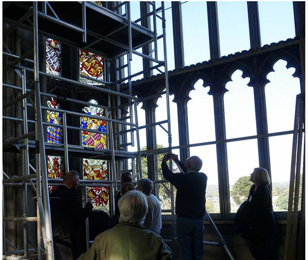
Figure 38: To agree the many details of EPG, including the treatment of the protective glazing itself, the most effective approach is to organise an on-site meeting with all stakeholders. This is particularly effective if it is possible to discuss in situ mock-ups of the proposed designs.
