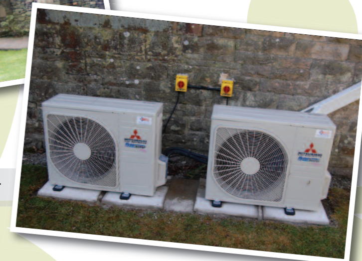
Air Source Heat Pumps at Mosser
